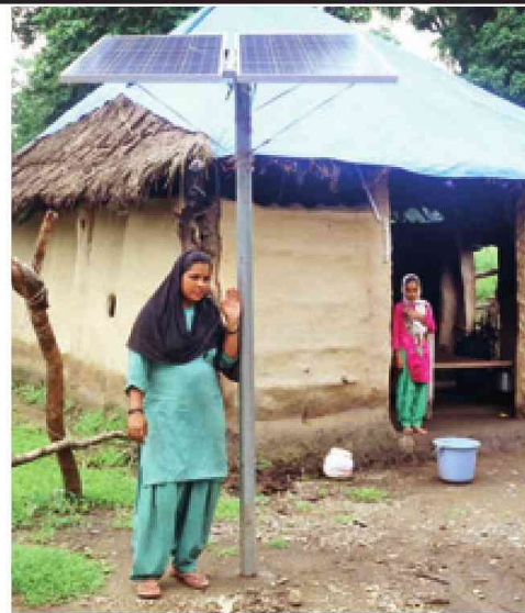
Haldu Khata and Jafrabad got their first fans and bulbs under Modi government's flagship rural electrification scheme, Deendayal Upadhyaya Gram Jyoti Yojana
