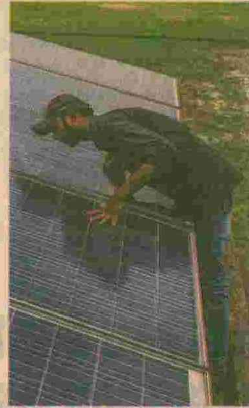
The current installed capacity of solar in India is around 20 GW
